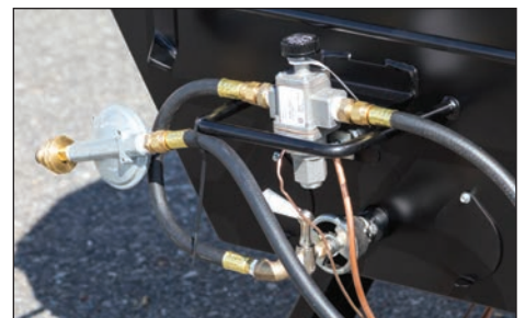
Gas Safety Valve
